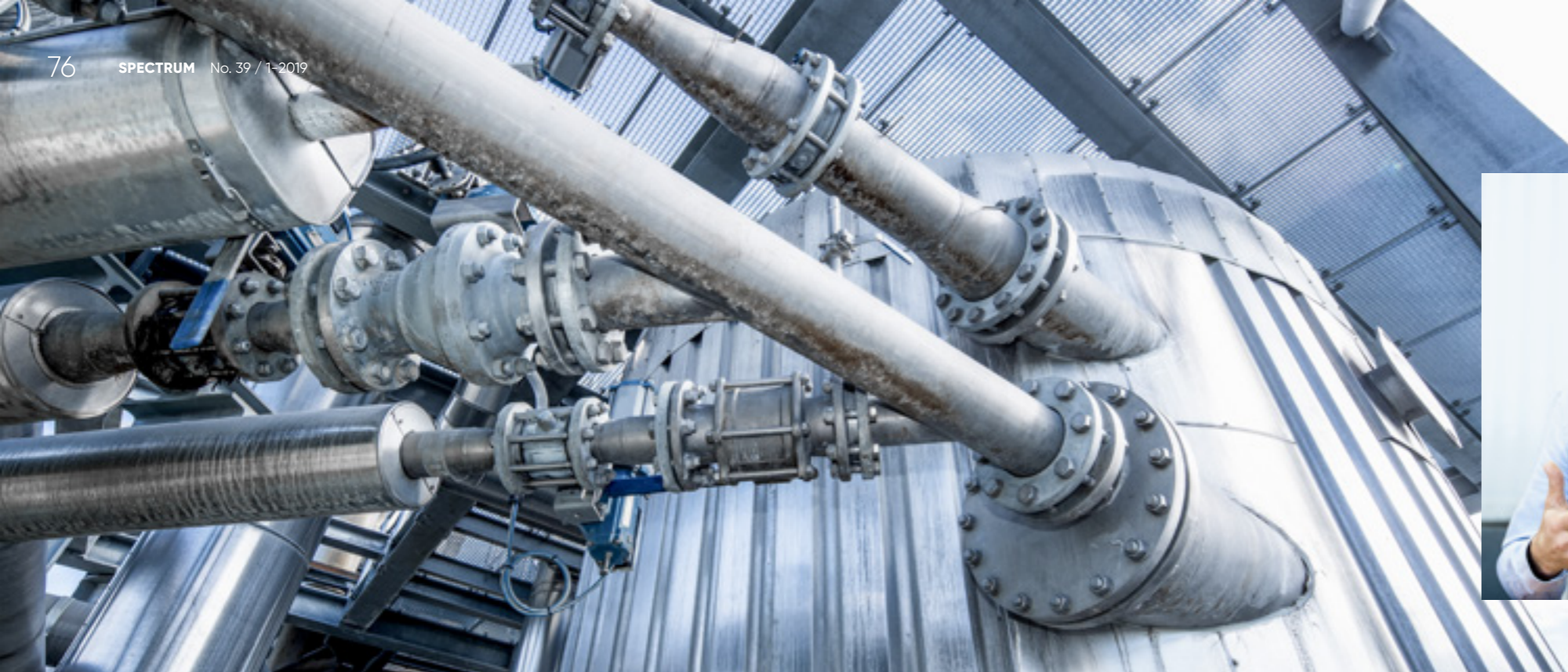
Black liquor is flashed in new ANDRITZ efficient flash tank utilizing FlashLance™-technology.
