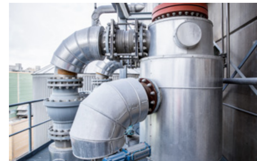
Impregnation liquor pre-heaters are part of the heat optimization system.
