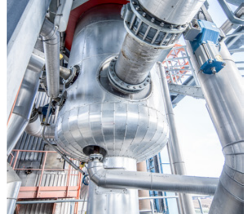
Vapor reboiler generates fresh steam utilizing the energy of hot black liquor (Flash steam) and fractionates the flash steam condensate to turpentine rich and clean condensates.
