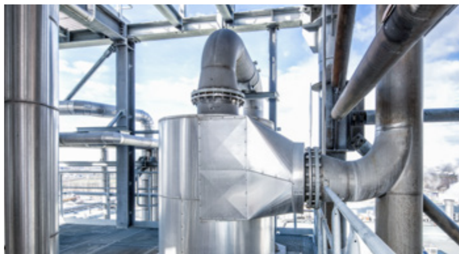
New gas handling system ensures safety and odour-free operation of the chip bin.
