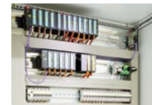
Tailored electrification equipment
