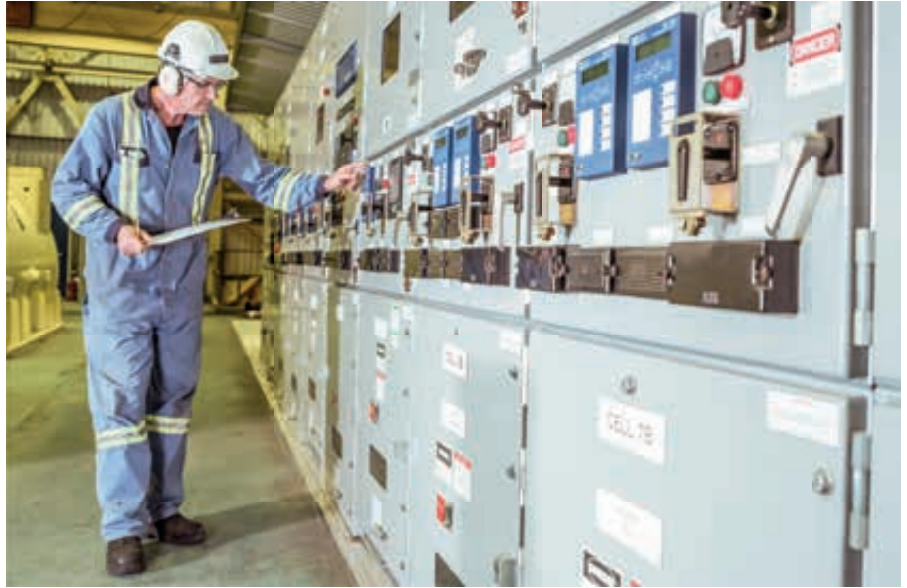
▲ Doug Tymos, Steam Plant Operator, checks the readings on a meter on the BUS-1 switchgear.
